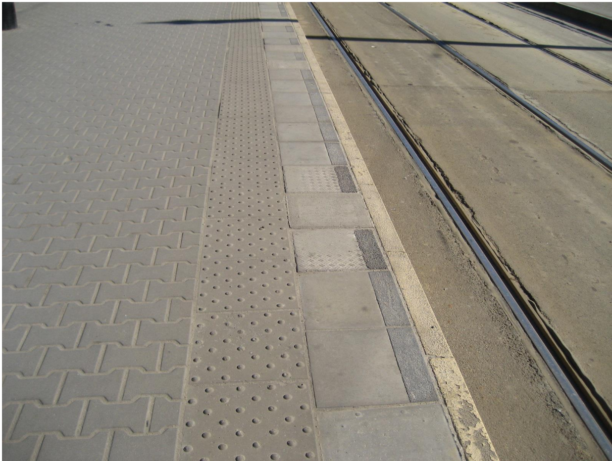
Figure 6. Example of improper maintenance of tram platform
